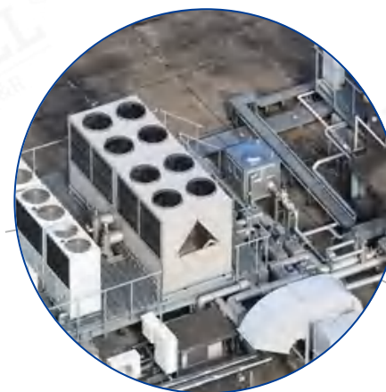
Building Ventilation System
