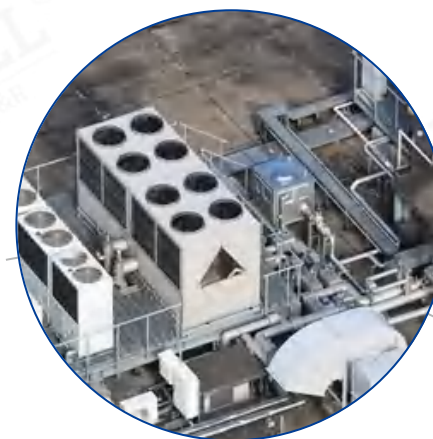
Building Ventilation System
