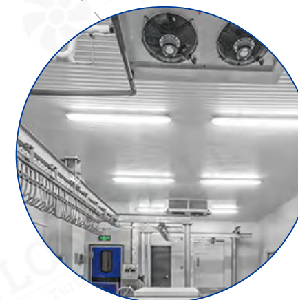
Workshop Ventilation System
