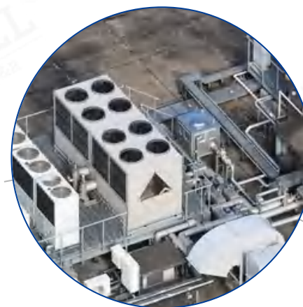
Building Ventilation System
