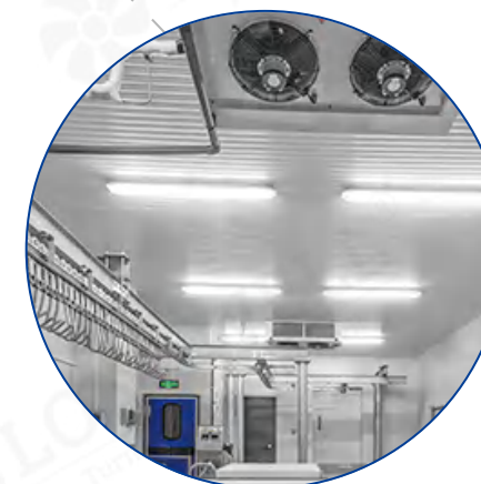
Workshop Ventilation System
