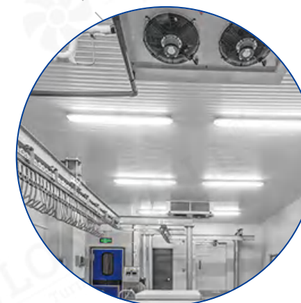
Workshop Ventilation System
