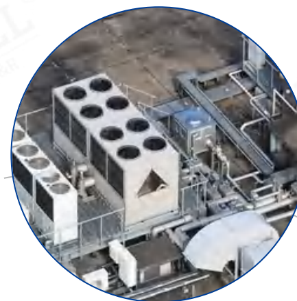
Building Ventilation System
